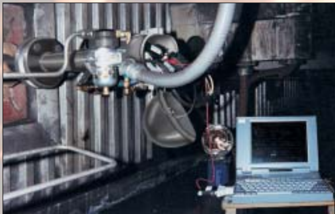
Infra-View ® Boiler Thermometer maintenance and customization being performed with a laptop computer in the field. Sensor programming can be accomplished anywhere along (2) wire loop or at DCS.
