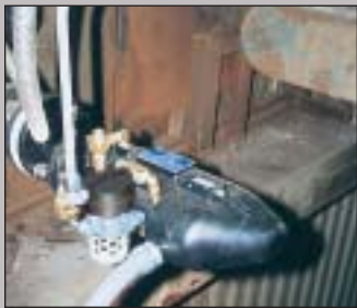
Infra-View ® Boiler / furnace Thermometer mounted on large coal fired utility boiler.
